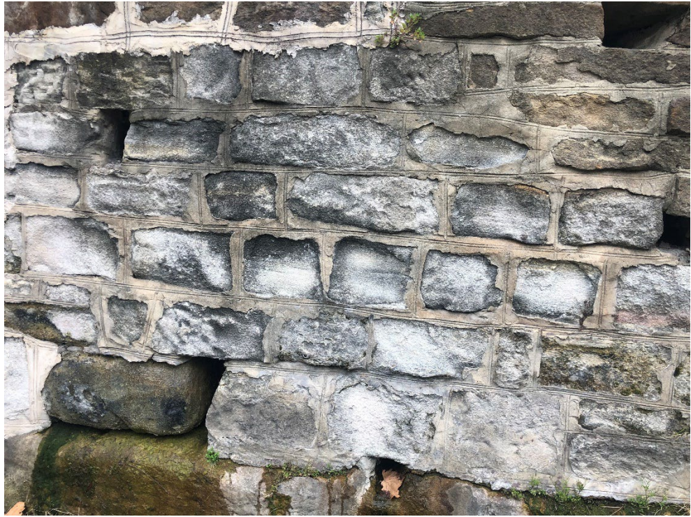
Figure 39: Detail of sandstone wall along Challis Avenue showing damaged caused by inappropriate pointing mortar.
