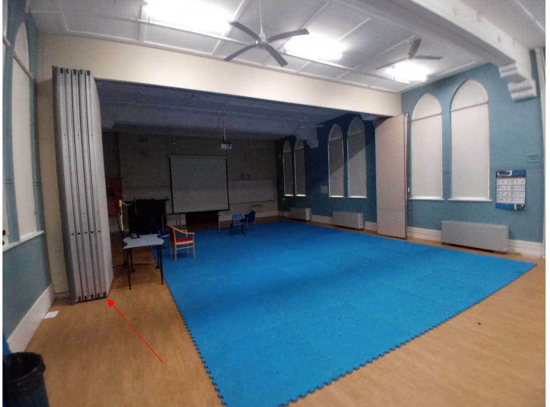
Figure 29: Two later (not significant) concertina walls to be removed from Mary Aikenhead Building B/C
