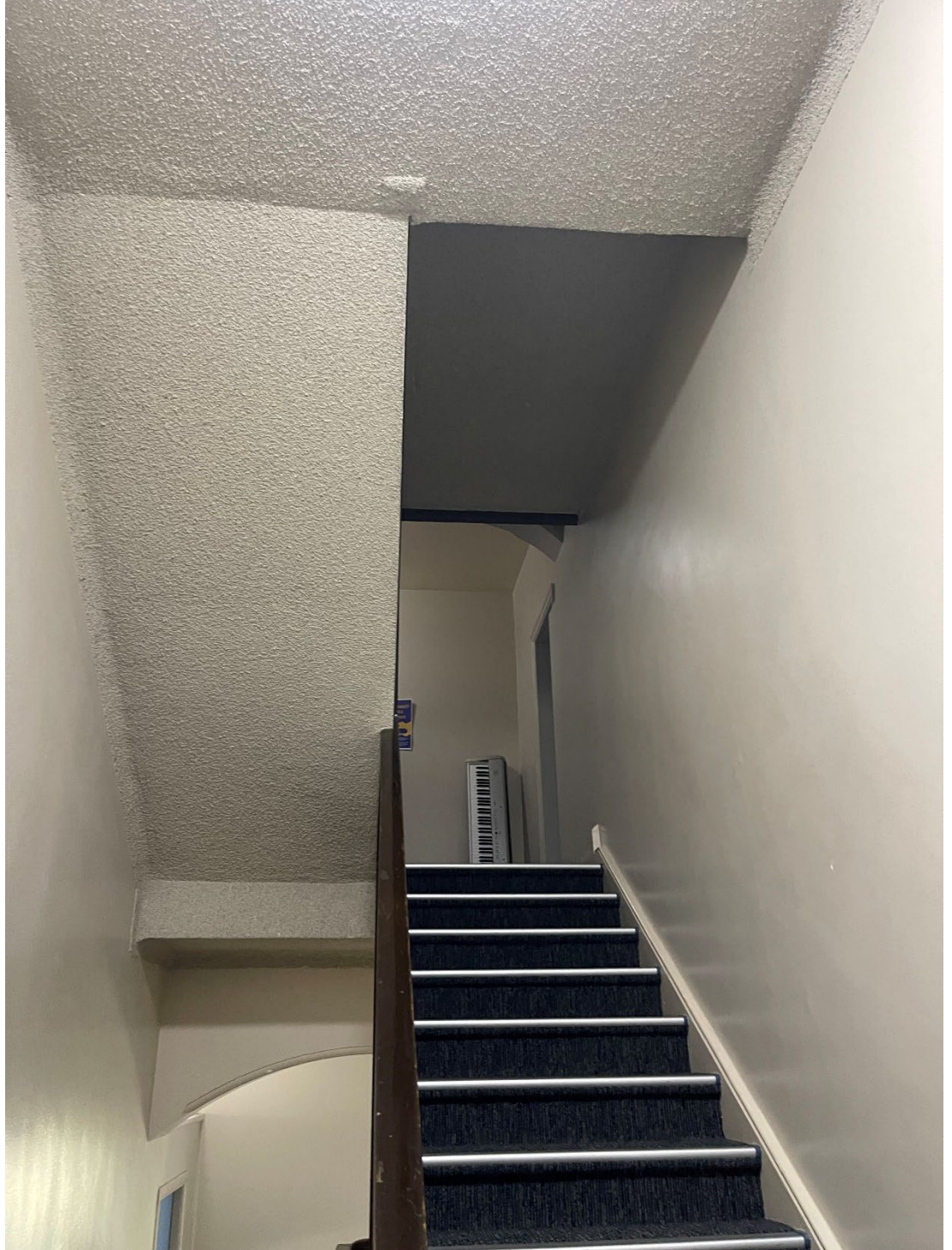
Figure 23: Rear stairs to be demolished to ensure new rear addition has level access to the Garcia building. Stairs have been altered with spray cement ceilings
