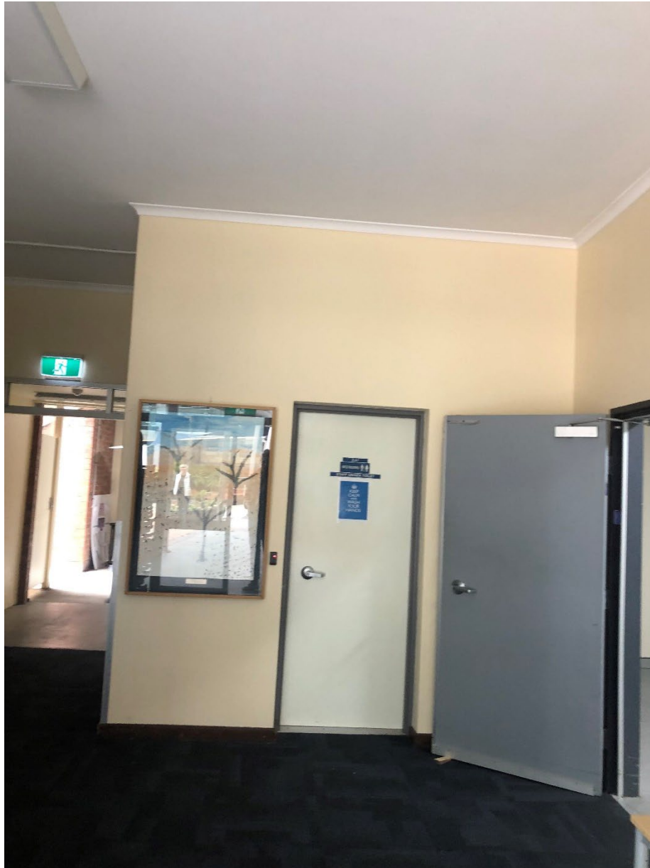
Figure 34: Internal view of chapel rear addition shown in Figure 32 above. These non-significant walls to be demolished.
