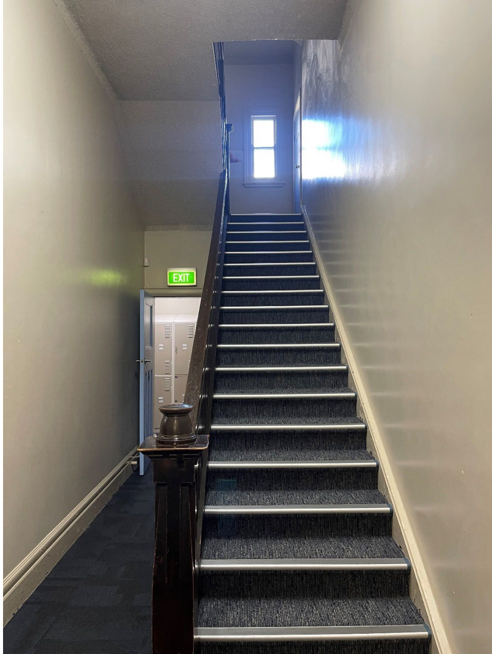
Figure 25: The rear stair balustrade does not display quality of craftsmanship shown in the front main building. This stair is proposed for demolition.
