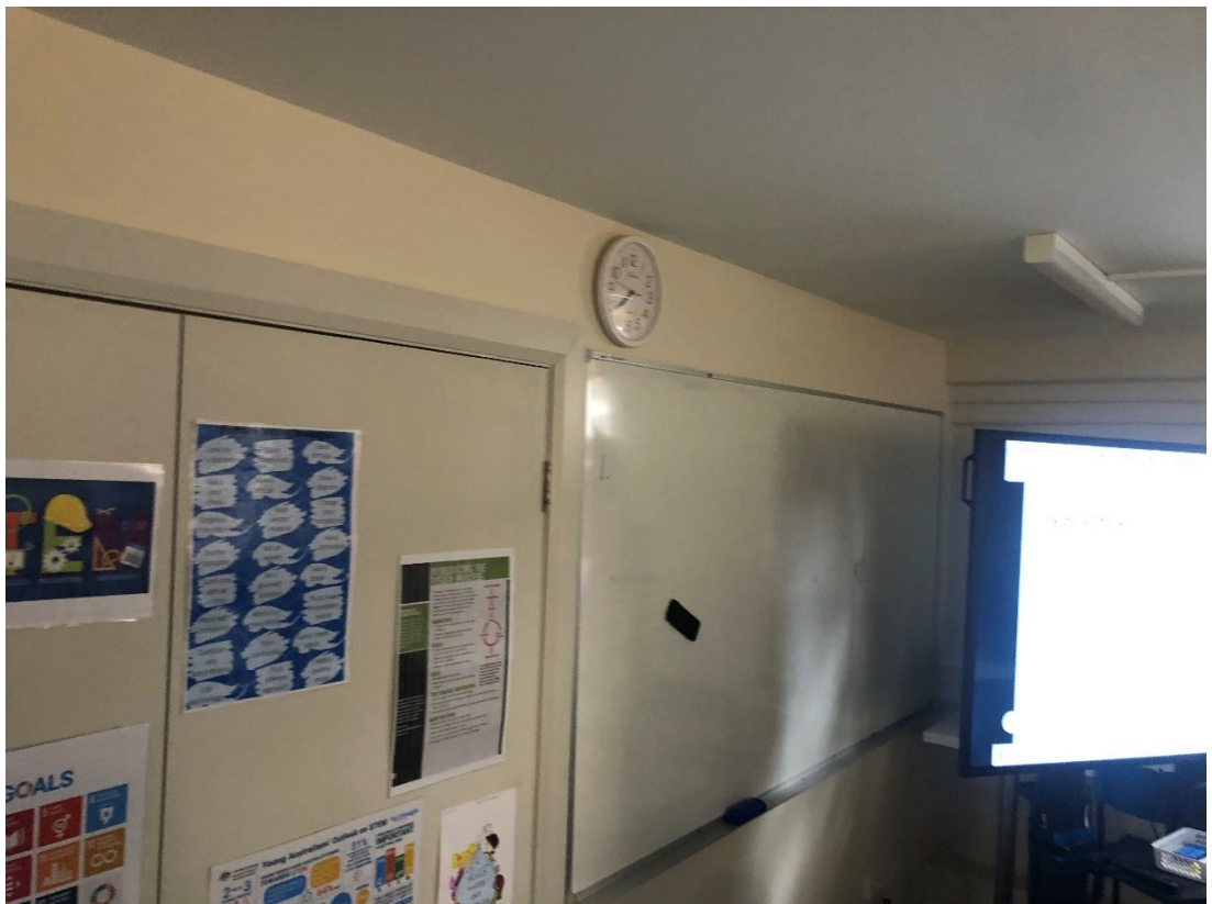
Figure 32: Second later gyprock wall to be removed in St Dominic's (Building A)
