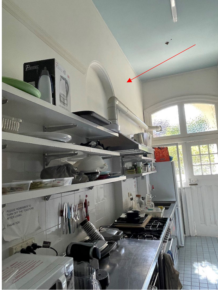
Figure 18: Wall on Level 3 Garcia to be removed. The original drawings show this wall has been previously altered. Refer to Figure 9 above.
