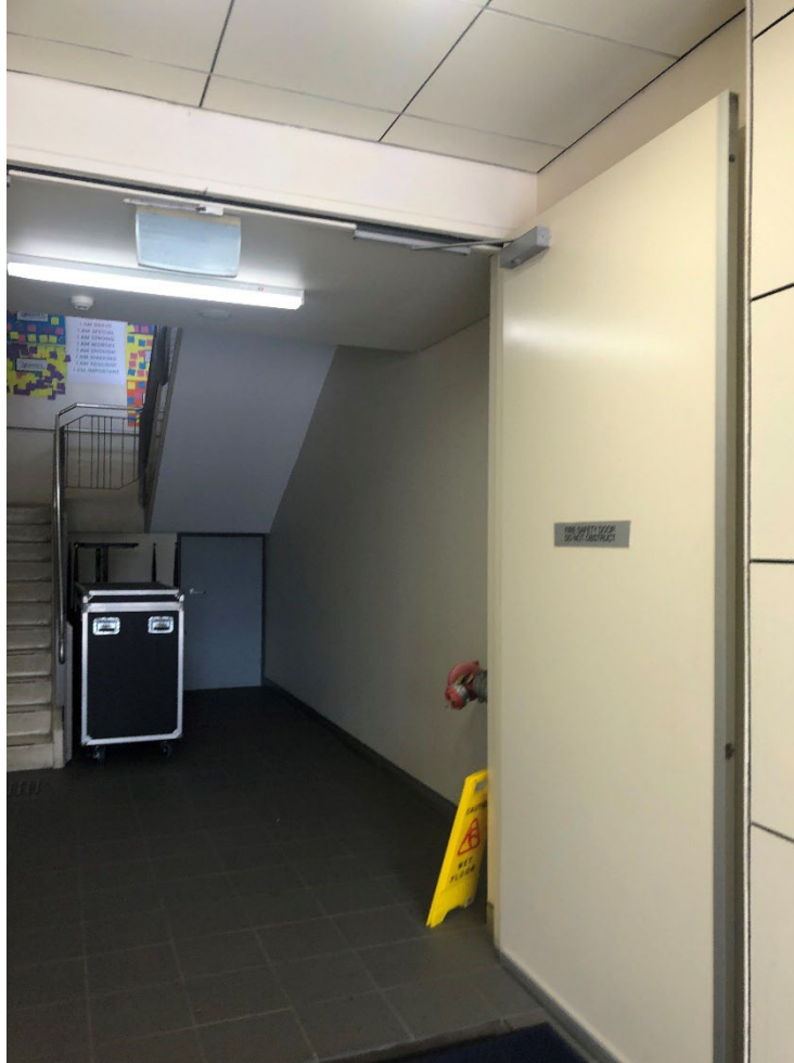
Figure 35: 1992 stair well walls to be demolished to improve connection of green spaces within the site
