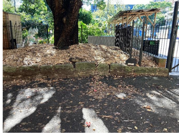
Figure 5. View of the sandstone garden edging to be separated from the northern side of APT16 by 600mm. (Source: CPH, May 2022)
